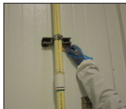
Condensation on walls, ceilings and behind pipes and conduit has been shown to promote Listeria establishment in the facility. Dripping to a concrete berm at the floor, especially if poorly grouted and sealed, can lead to intrusion of insulation and long-term reservoir for periodic contamination.
