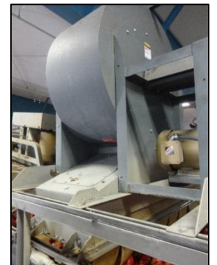
Out of reach equipment
