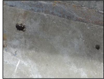
Holes from equipment that has been moved should be sealed to avoid harborage areas
