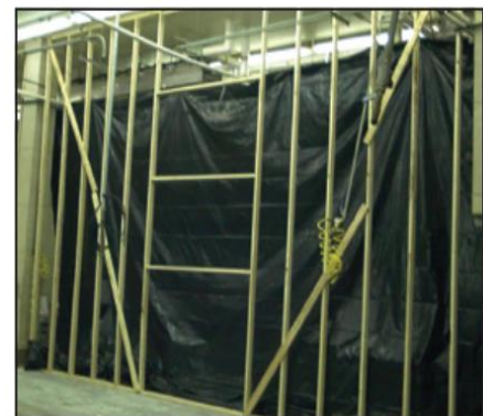
Temporary barriers can protect the production environment from aerosols and traffic that may carry Listeria exposed during construction.
