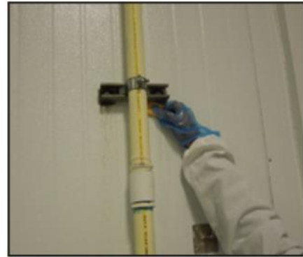
Condensation on walls, ceilings and behind pipes and conduit has been shown to promote Listeria establishment in the facility.
